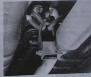
19.9B ...and ensure that the exhaust system mountings are in good condition
