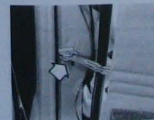
16.3 Door check link retaining pin and clip (arrowed)
