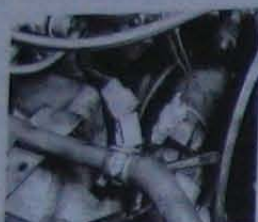
31.21C ...and the various other electrical components
