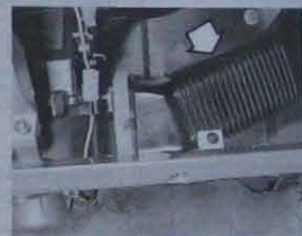
11.7 Blower motor to heater unit duct (arrowed)
