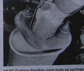
19.9C Tighten flexible joint nuts so springs are well compressed but are not coil bound
