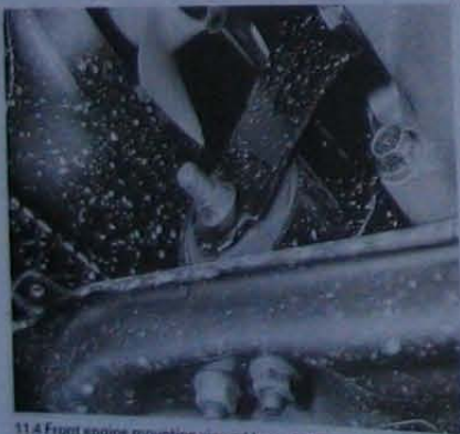
11.4 Front engine mounting viewed from underneath
