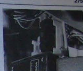
11.10 Blower motor circuit breaker is located directly above the circuit fuse box
