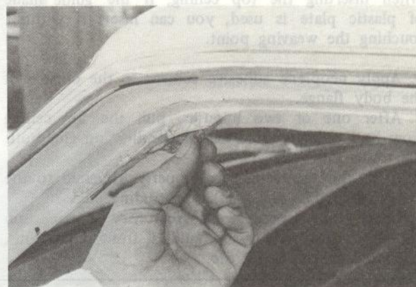
Fig. 14-105 Tearing of ceiling cemented surface
